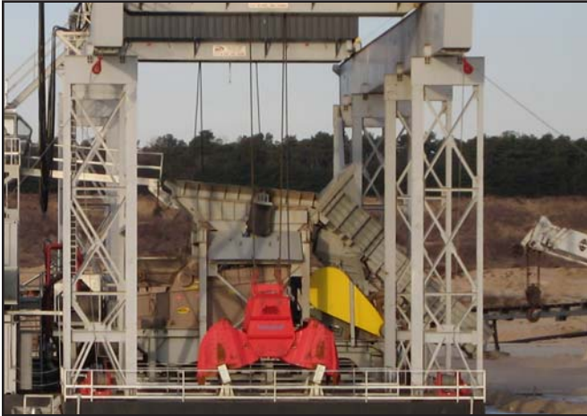
Winches are mounted at each corner of the barge. Lines are run to snatch blocks overhead and connect to anchors on shore.
