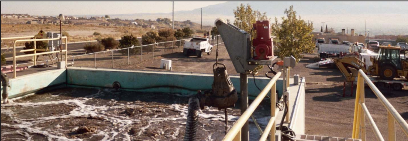
A 4771 installed at a pump station helps with routine maintenance on the pumping equipment.
