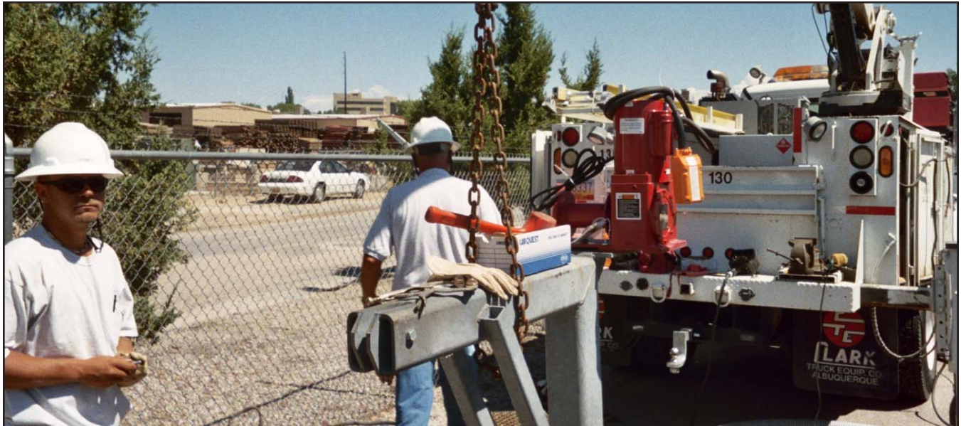
Workers prepare a Thern 4771 electric winch for installation at the Rio Rancho Water Utility facility.
