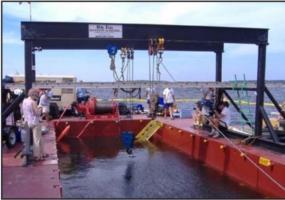
Above: The crew prepares the equipment; including the Thern TA series BIG RED air winches, for the lift.
