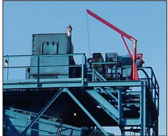
A Thern model 571 davit sits atop a transfer tower.
